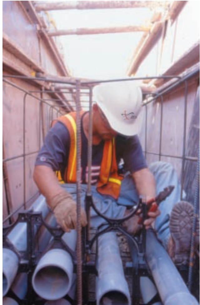
Photo courtesy of Integrated Electrical Services, Inc.
